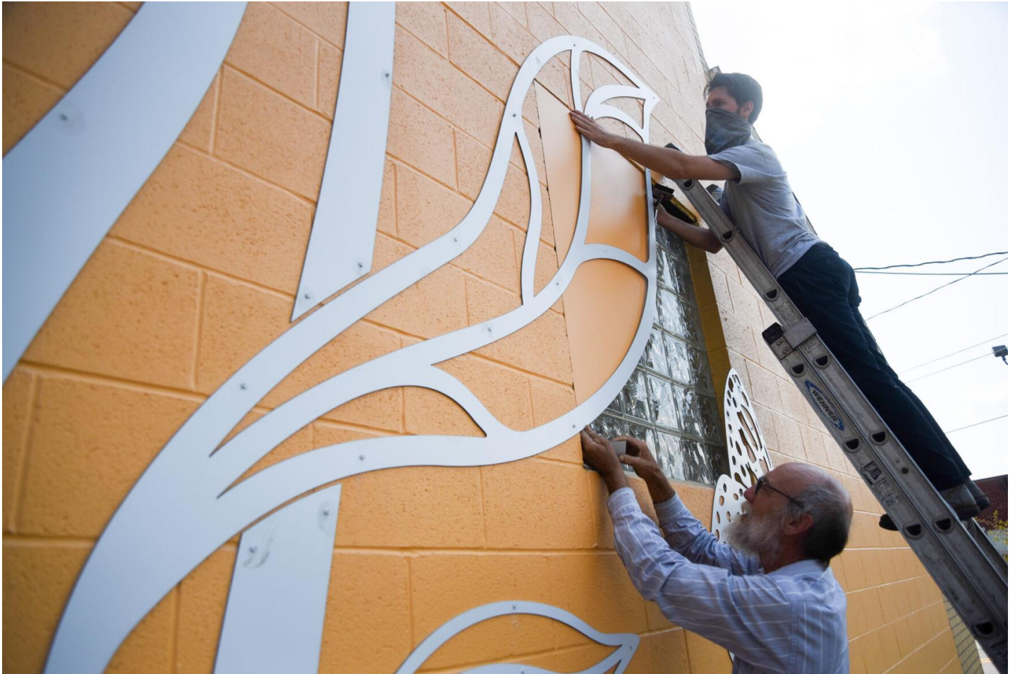
Local artist Doug Lodge (left) and Lee Scandinaro install backing to a section of a large metal mural on the Snodgrass Building on Wednesday afternoon.
